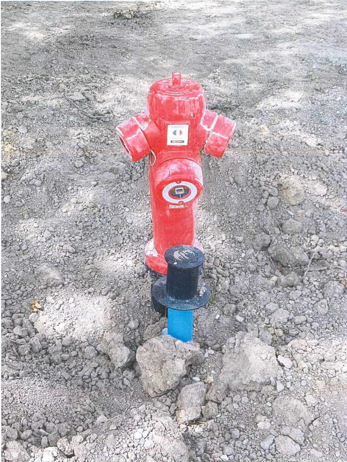
Poteau incendie privé - MENUT ST CYR-EN-VAL
